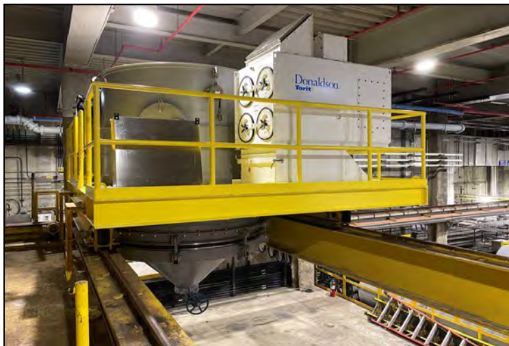
Carbon Loading and Dust Collection System
