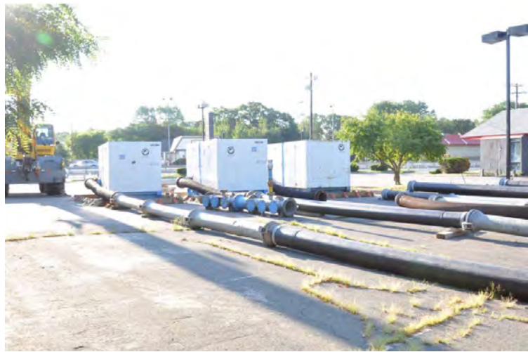
Figure 2: Bypass equipment at Junction Chamber No. 1
