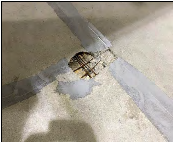
Existing Cracks and Voids in Floor
