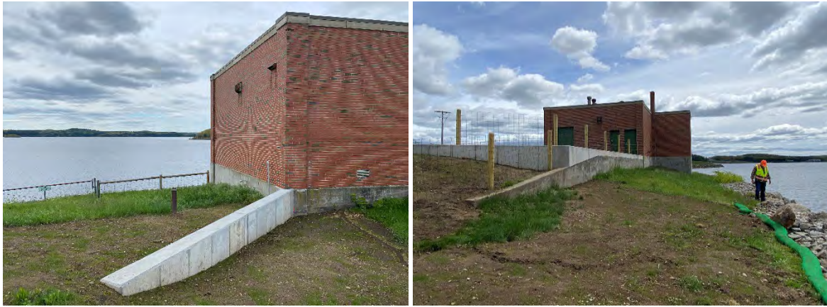
Figure 1. Parapet walls east and west reconnect the North Dike at Leominster Pump Station
